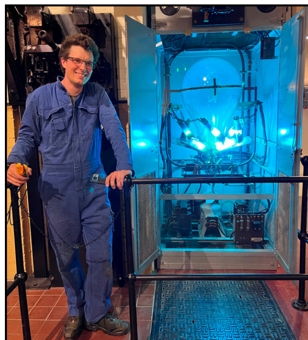
Volunteer Ben next to the Arc Rectifier in the Electric House.
