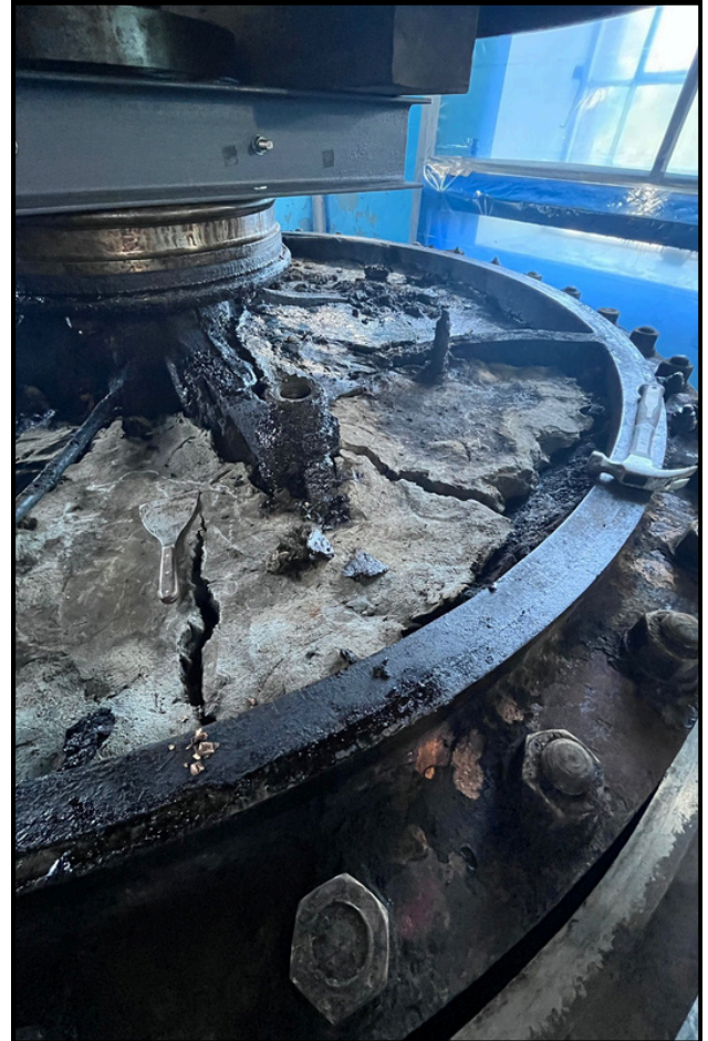
Asbestos inside the 90 Inch Engine cylinder.
