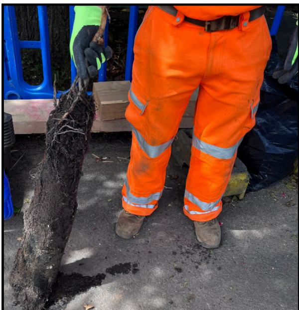
The blockage of tree roots that was pulled out from the toilet pipe.
