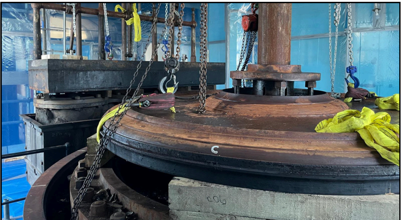
The 100 inch false cover on timber chocks with the valve box cover behind.
