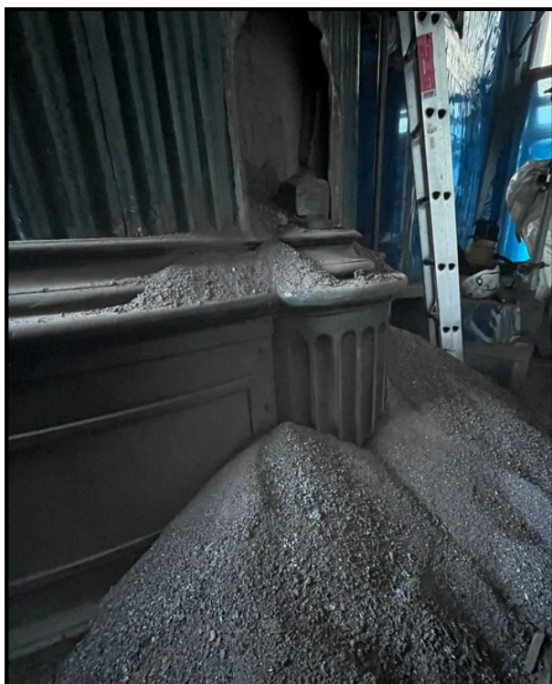
The material that fell out of the cylinder when the lagging sheets were removed.
