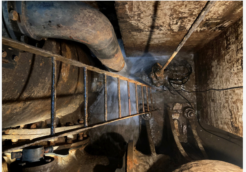
Overflow from engine suction surge vessel back into basement underneath the Bull Engine.
