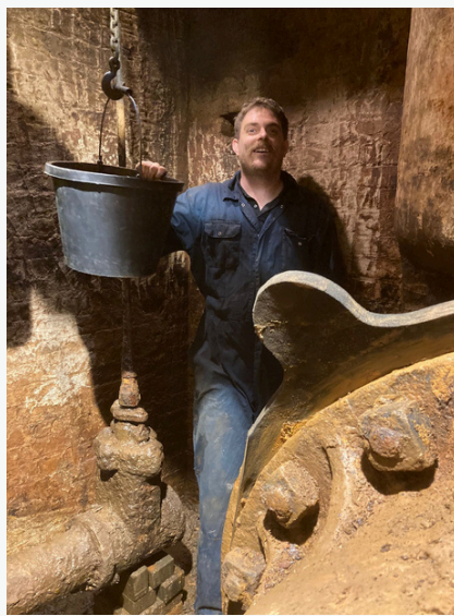
Figure 11: Glen Williams volunteer staff removing rust debris from basement floor of Bull
