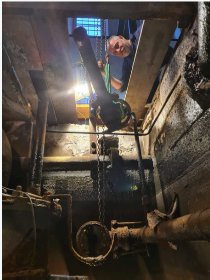
Figure 7: Richard Albanese lifting out condenser cooling water valve from condenser tank on B&W
