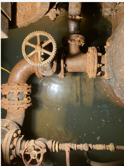
Figure 10: under bull- start of works in basement pumping out water to Bull
