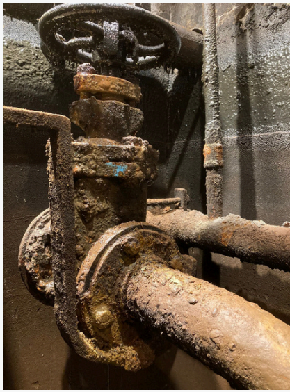
Figure 5: inch water pipe joining 3 inch water pipe and condenser cooling water valve to B&W
