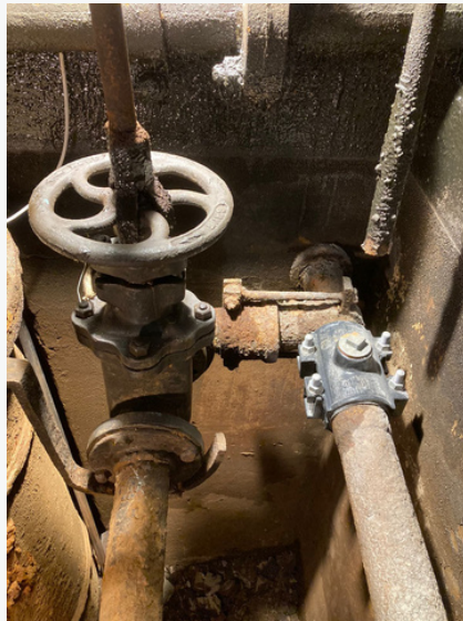
Figure 8: Condenser cooling water valve overhauled and reinstated. fractured 1 inch connection hole entombed under new Viking Johnson repair clamp
