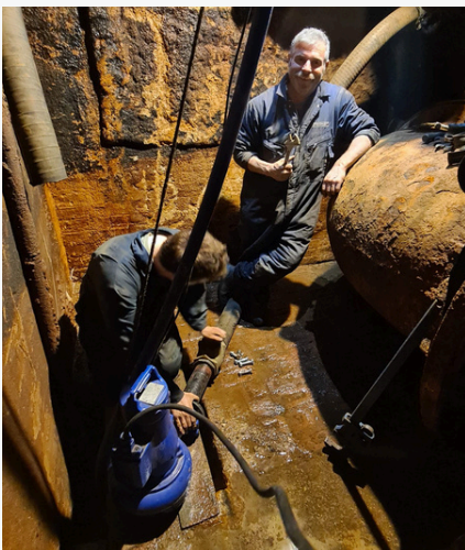
Figure 13: bull engine Glen Williams and Richard Albanese installing JST submersible pump to Bull
