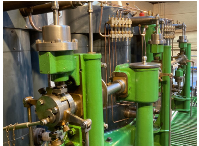
Valve gear at the top of the Triple Expansion Engine.
